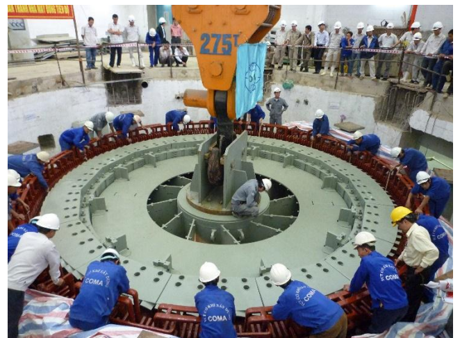
Song Tranh hydropower project
